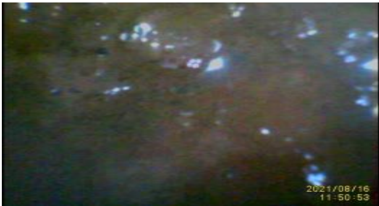
Fig. (5): View of internal wall of secondary circuit pipe of TRICO II reactor after visual inspection with the multifunction video KC350
