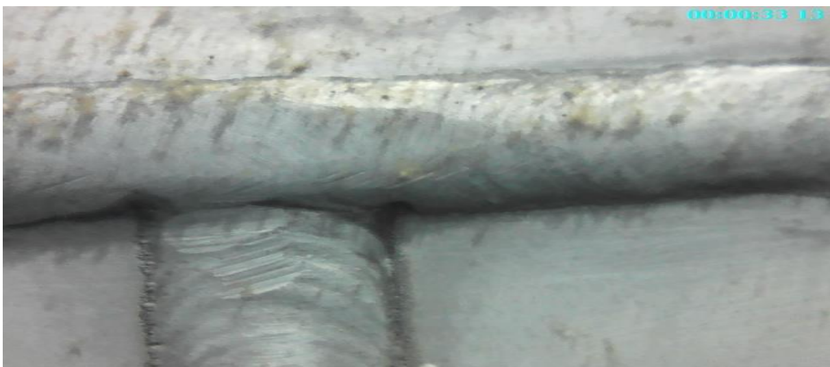
Fig. (5): Photo of good welds in T: horizontal weld (CH2) and vertical weld (CV2). The photo was taken with the underwater endoscope USB 2.0.
