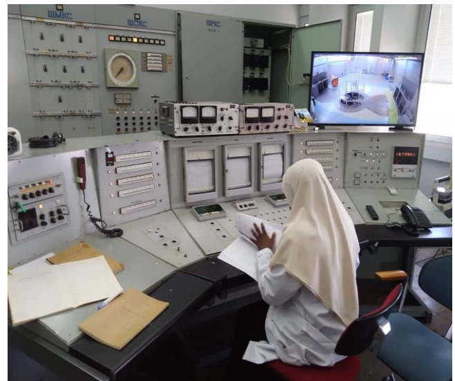
Fig. (3): Control Desk of Critical Facility
